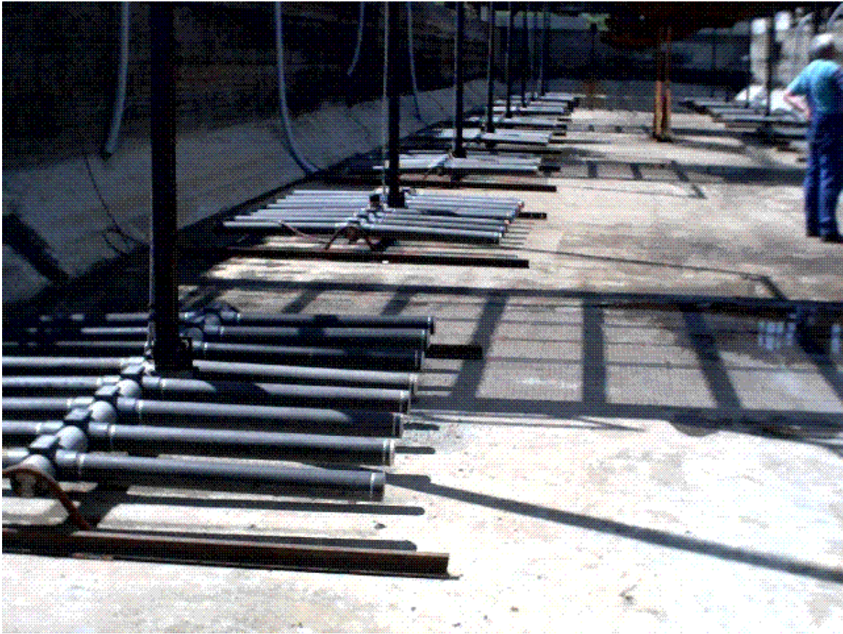
Sample Tube Diffusers at the bottom of a Sewage Treatment Tank
